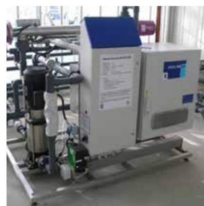
Figure 4.0 Adequate disinfection equipment is needed to prevent discharge of nutrient solution from mineral wool crop-growing systems and hence obtain a fertilizer use efficiency of (almost) 100%. The photograph shows one of the possibilities, disinfection by ultra-violet radiation. http://www.hydroponics.com.au/disinfection-methods-an-australian-perspective/
